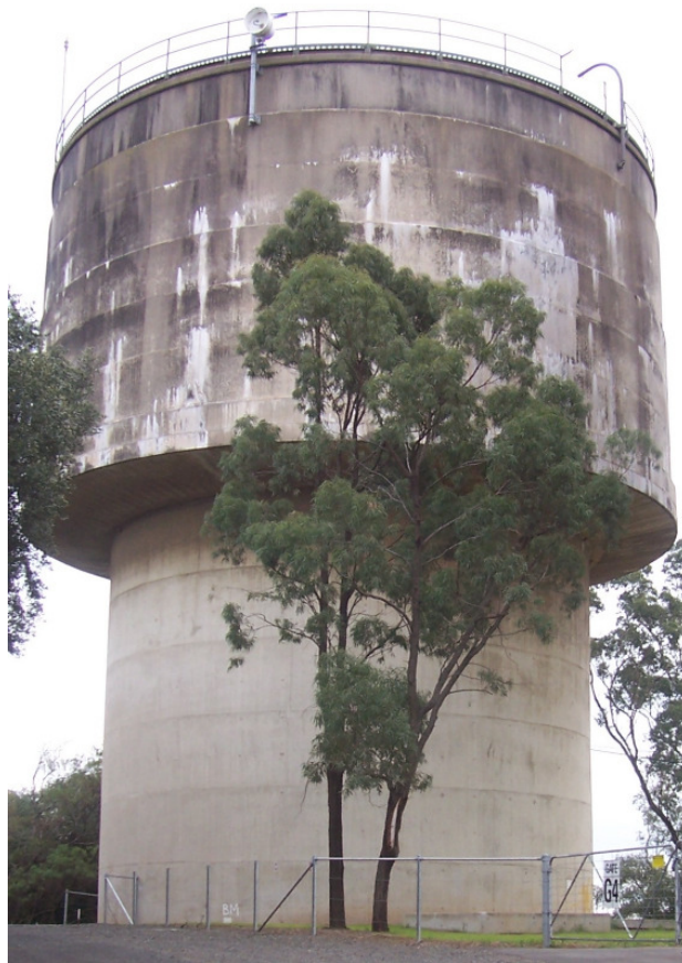
Figure 8 - Concrete wineglass tank, 2ML storage capacity
